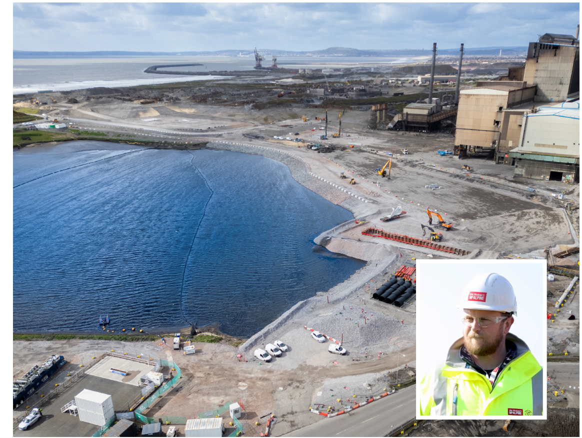
A massive engineering operation has changed the face of the steelplant lagoon. Inset: Johnathan Lewis
