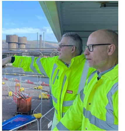
Sir Robert McAlpine's Paul Bird (left) points out the progress being made on the enabling works for the EAF at Port Talbot
